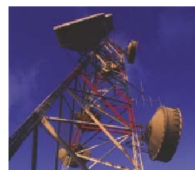
A typical Neos wireless microwave installation
