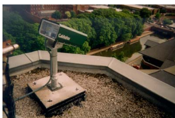
100Mbps Data link installed for major financial institution, connecting remote offices in Reading, UK. Installed 1998.
